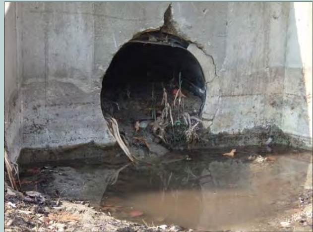
Debris and foreign material from an existing pipe draining into a retrofitted detention basin.
