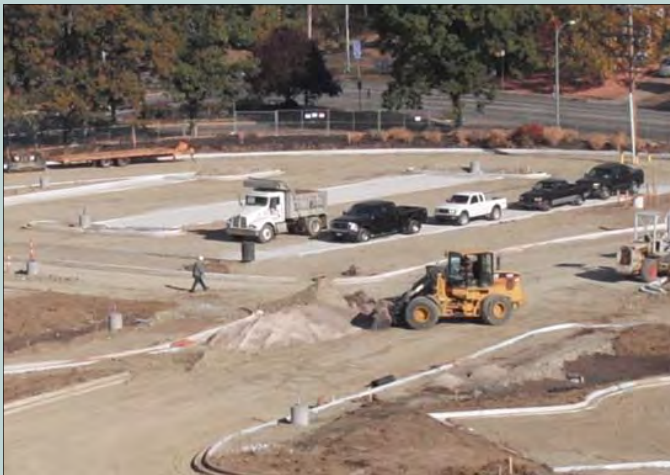
Stock piled raw materials adjacent to the porous pavement areas under construction, vehicles parked on features.
