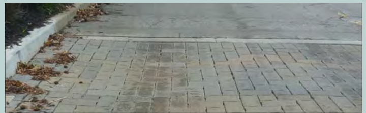
Rutted porous pavers from heavy traffic.
