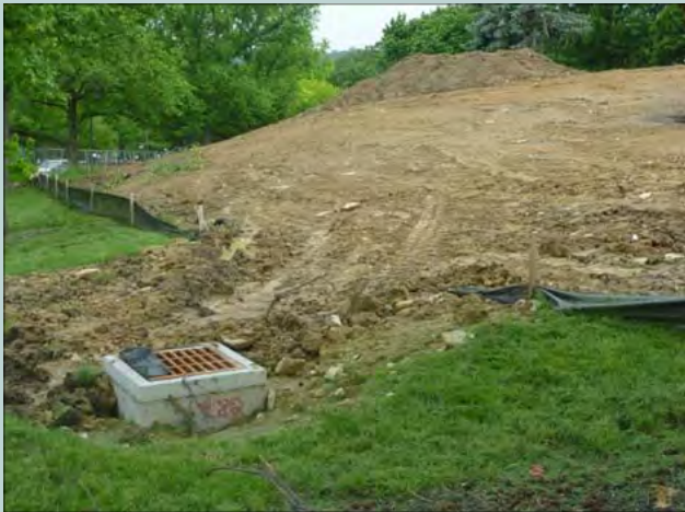
Broken silt fence promotes erosion and sediment build up in the proposed green feature.
