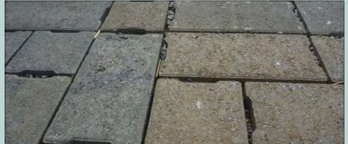
The pea gravel in this system has settled.
