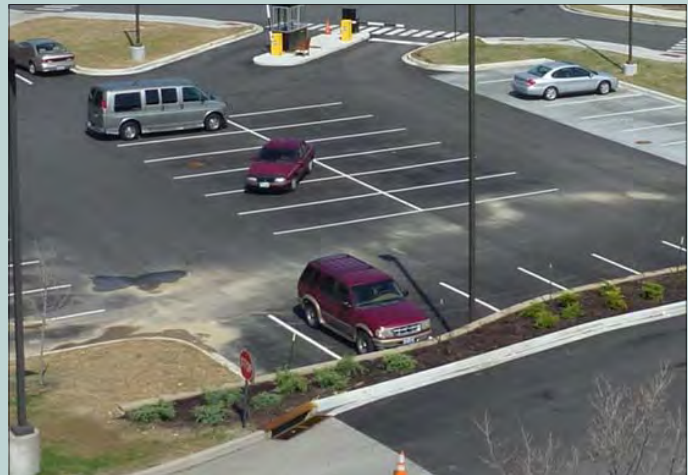
Excess silt and sediment on the porous pavement surface can prematurely clog the system.
